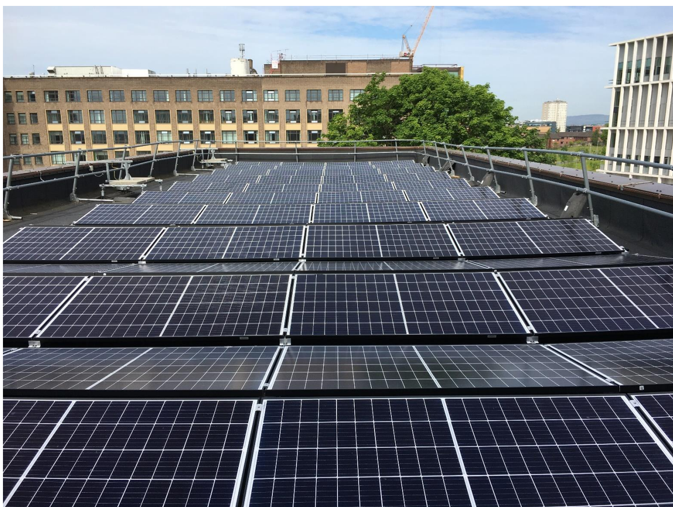
Solar panels on the roof of the Sir William Duncan Building, part of a 0.5MW deployment underway
